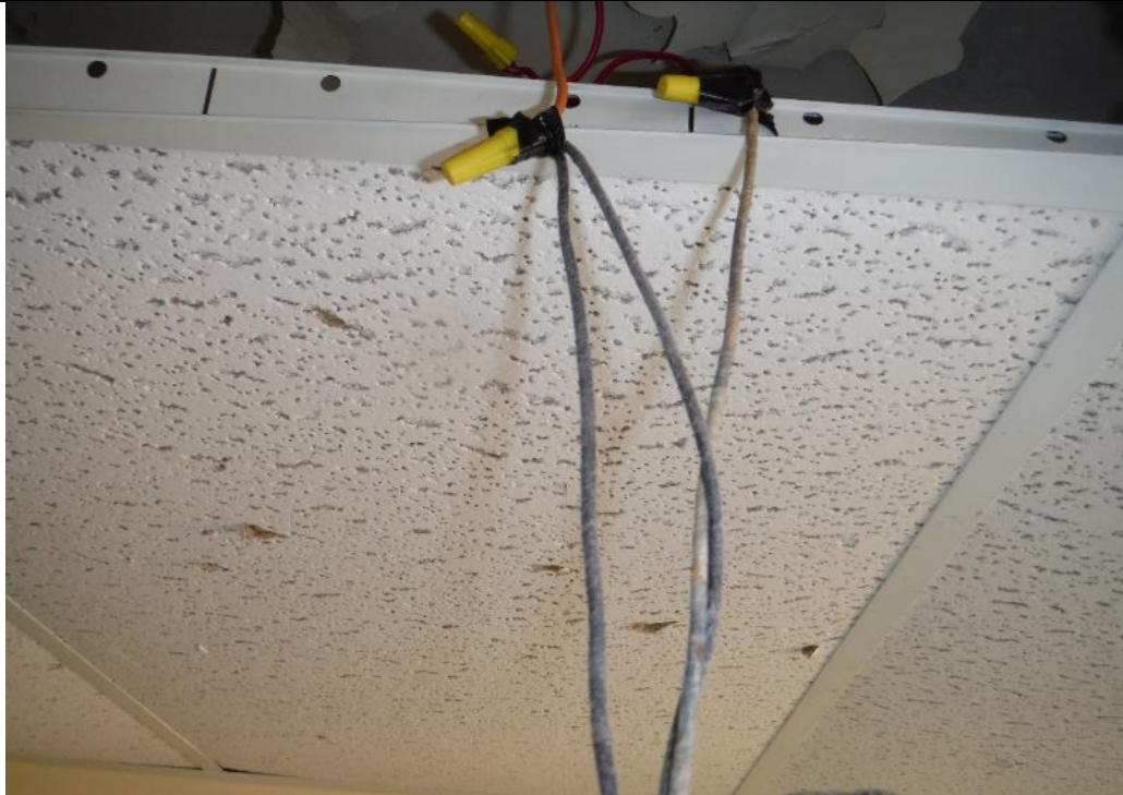
Samples 58 – 59 Electrical Wire Insulation on wires coming from Ceiling Lights
