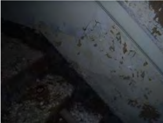
Stairwell Showing Paint Chips on Floor
