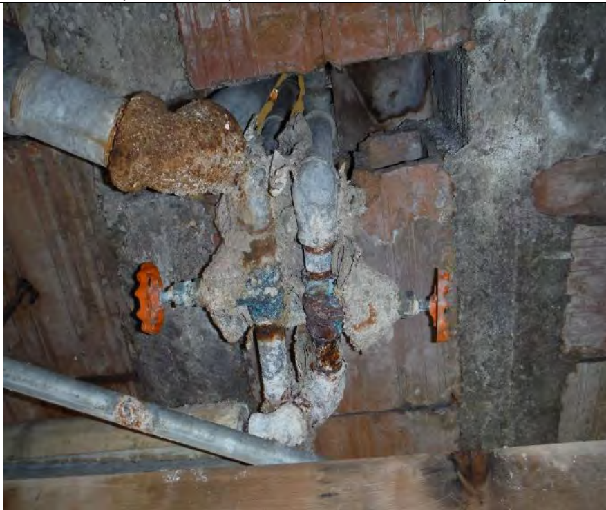
Samples 36 – 38 Mudded Fittings. Example of poor condition of fitting
