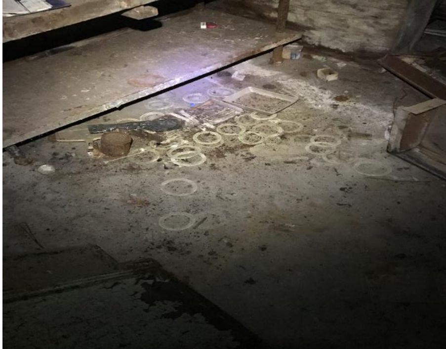
Samples 145-147 Boiler Gaskets covering the floor
