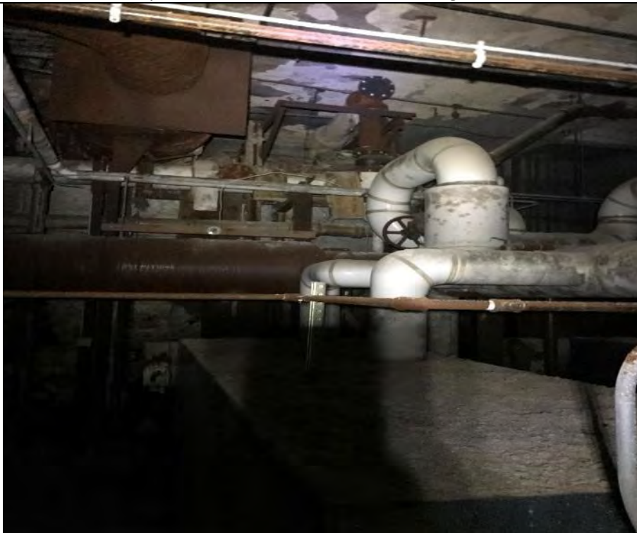
Samples 151-153 Muddied fittings and Asbestos Debris throughout
