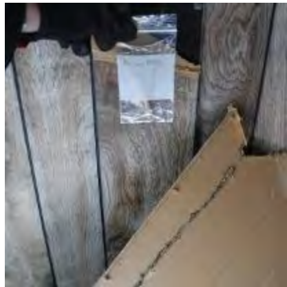
Warden 47 – Wall Mastic
