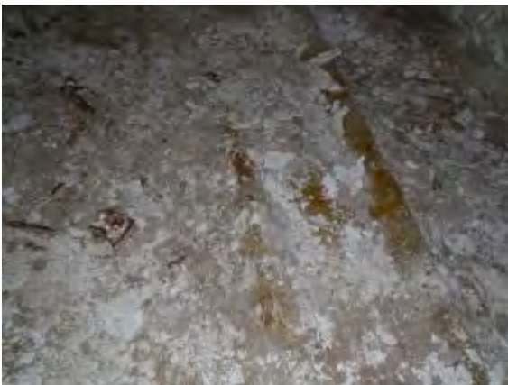
Paint Chips Covering Floors
