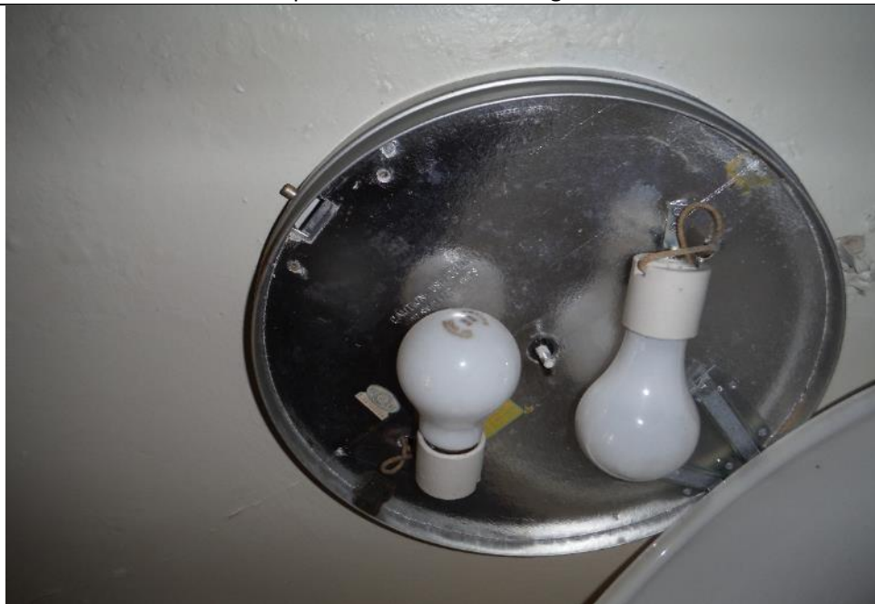
Sample 57 Heat Shield on Circular Lights on the ceilings and Wire Insulation
