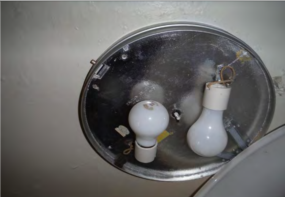
Sample 57 Heat Shield on Circular Lights on the ceilings and Wire Insulation
