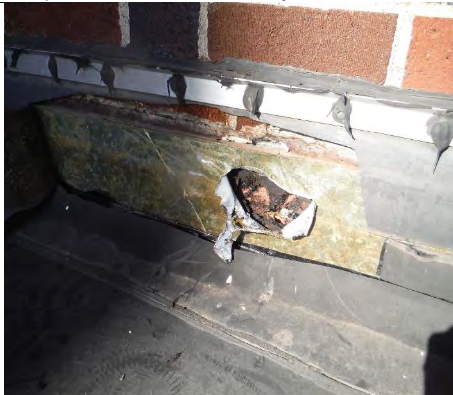
Samples 13-15 Parapet Wall Flashing – Black Tar Sample 18 - Silver Caulking Above Black Tar
