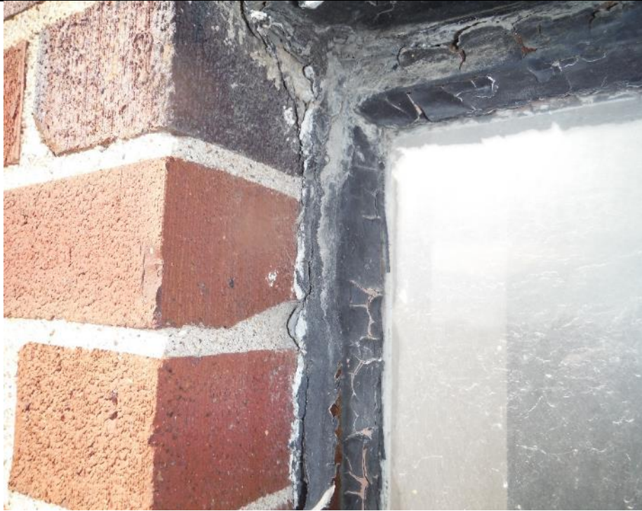
Samples 10-12 Window Frame Black Caulking between Brick and Frame
