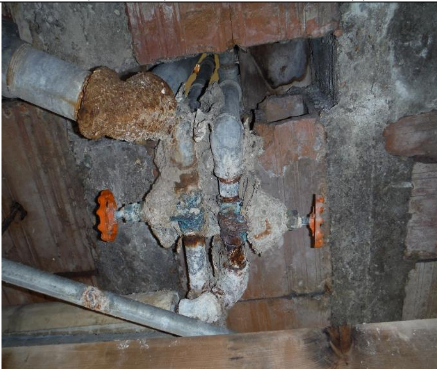
Samples 36 – 38 Muddled Fittings. Example of poor condition of fitting
