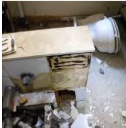
E BLDG 40 – Bathroom Tile Mastic
