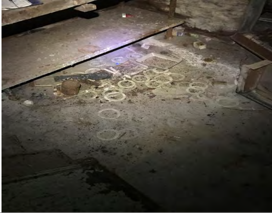
Samples 145-147 Boiler Gaskets covering the floor
