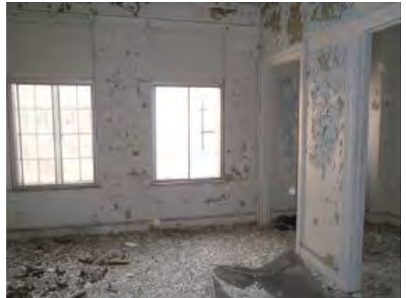
General Condition of Paint and Substrate
