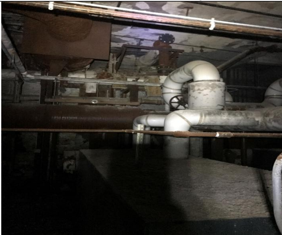
Samples 151-153 Mudded fittings and Asbestos Debris throughout
