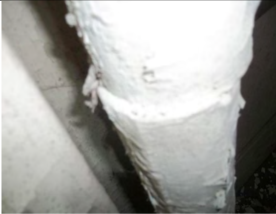
Samples 39-41 Air Cell Pipe Insulation on 2" Straight Pipe
