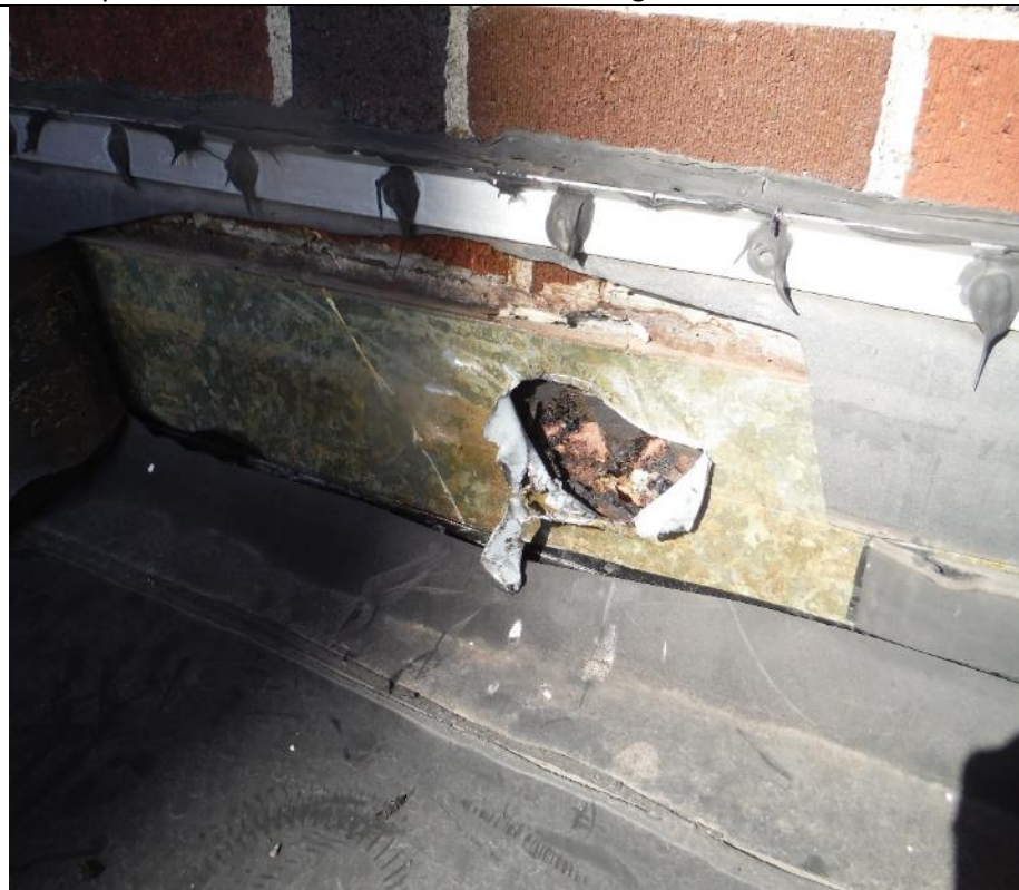
Samples 13-15 Parapet Wall Flashing – Black Tar Sample 18 - Silver Caulking Above Black Tar
